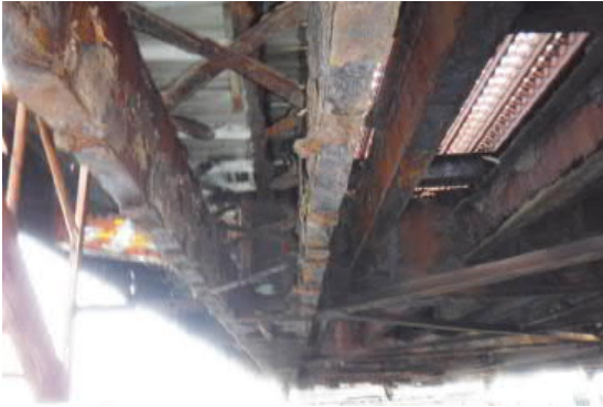
Image 3: Severe Deterioration and 100% Loss of Lattice Bracing in the Swing Span Lower Chord
