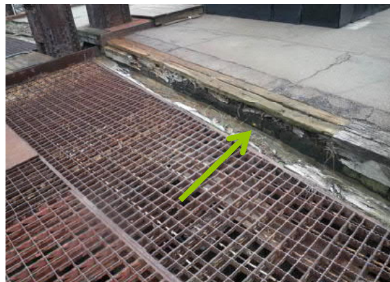
Image 7: Vertical Alignment Differential between the Swing and Approach Span
