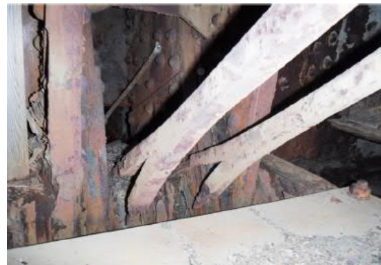
Image 6: 100% Section Loss of Eye Bars Diagonals in the Swing Span
