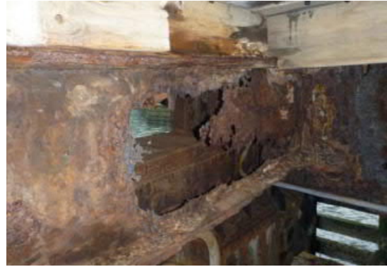
Image 2: 100% Section Loss in an Approach Span Stringer
