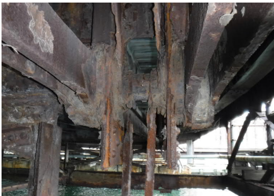
Image 5: Severe Deterioration of the Verticals Below the Deck and Pin
