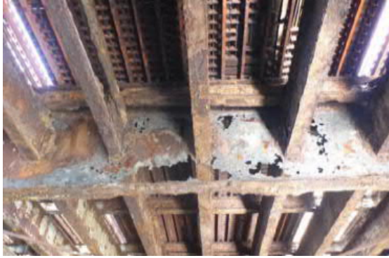
Image 1: 100% Section Loss in a Swing Span Floorbeam
