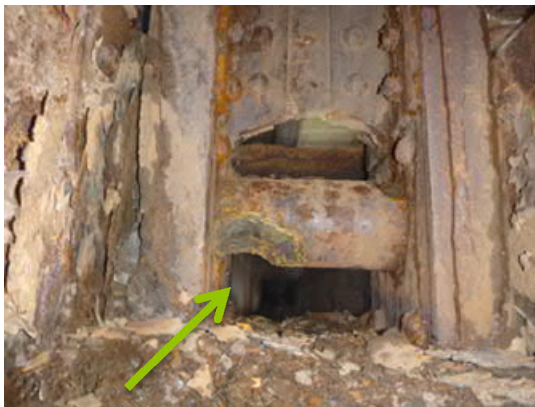
Image 10: Deterioration of the Pin
